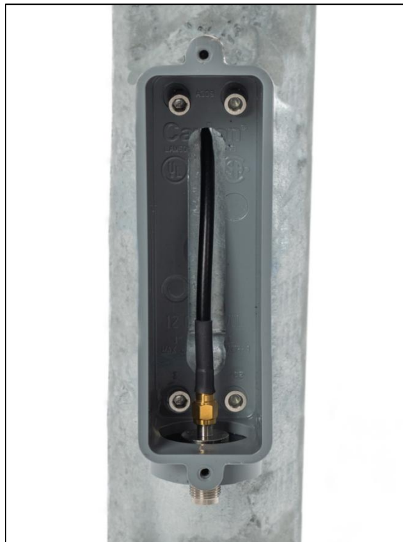
Figure 10: Junction box with SMA cable connected
